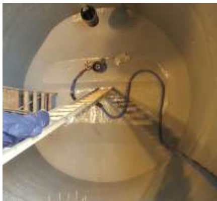
Typical Polyurethane epoxy finished, Pump Well.
