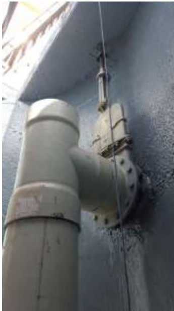
Typical isolation valve installation, Pump Well.
