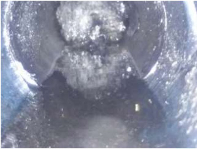
Pump inlet pipework blockage
