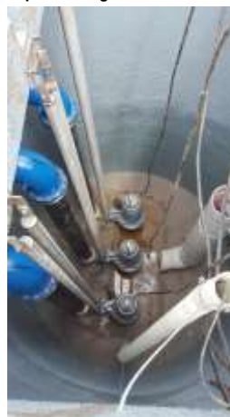
Typical triple railed guided duck foot pump installation.
