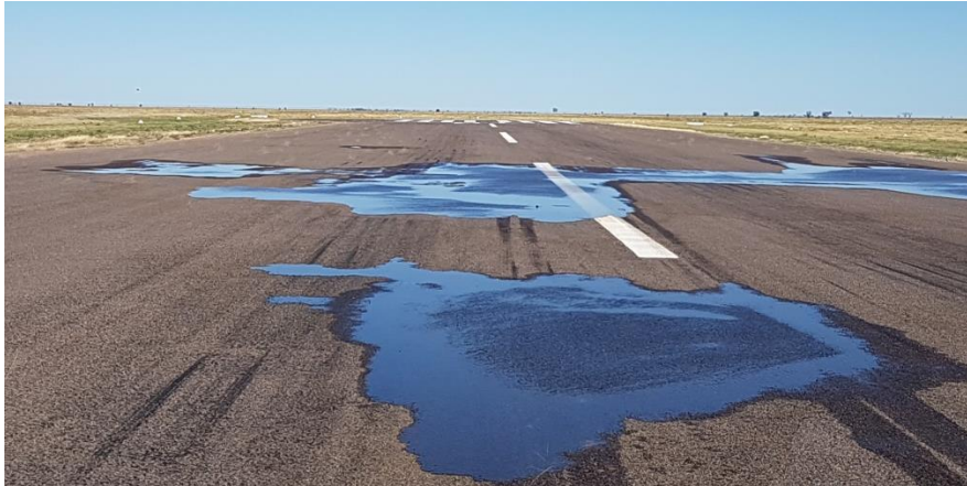
Figure 1 Ponding at west end (touch down area)
