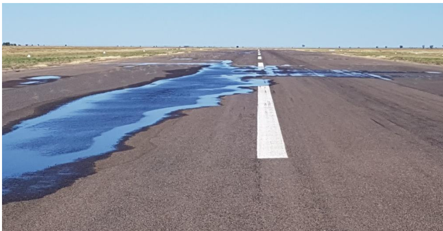
Figure 2 Ponding near centre of runway
