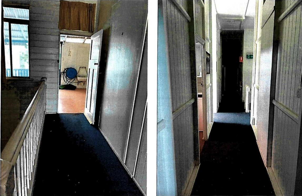
Figure 4-9 Condition of the Upstairs Area
