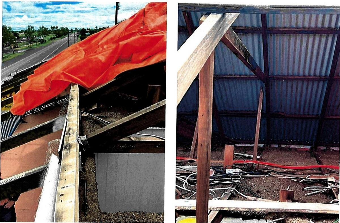
Figure 4-22 View of the tie downs and failed truss
