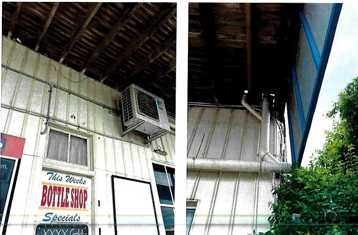
Figure 4-12 Condition of the external West wall (left image) and a deteriorated column in the South-East Comer (right image)
