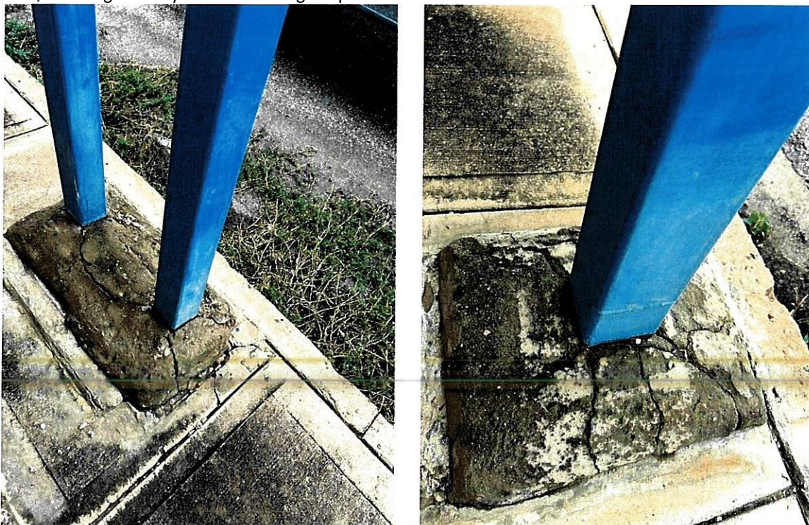
Figure 4-19 View of the spalling concrete footings and corroded steel columns
