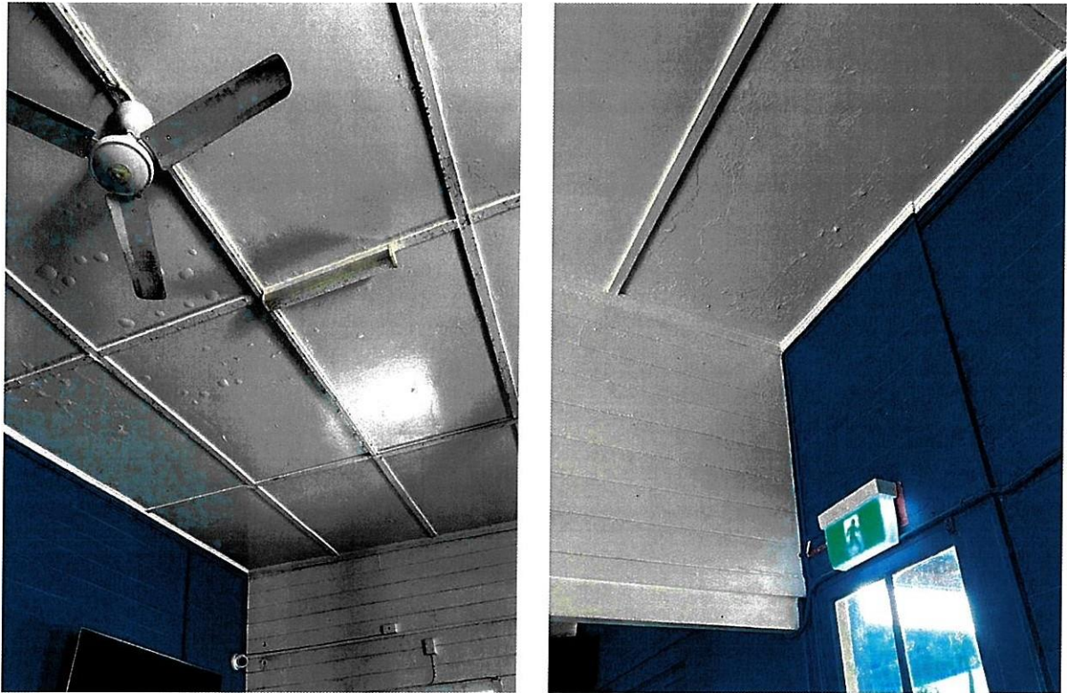
Figure 4-6 Water Ingress evident in the ground floor ceiling
