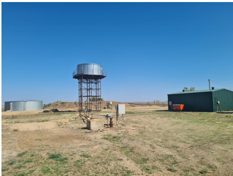
Figure 2.6 - Photo of Kynuna Bore and Elevated Storage Tank
